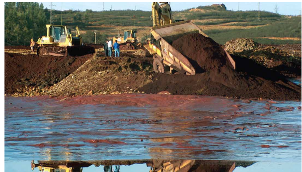
Full sludge pond with very low shear strength
