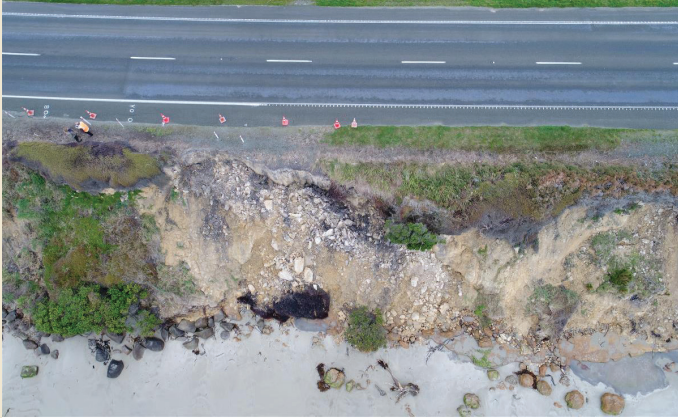
Road cracking & coastal erosion before the project commenced
