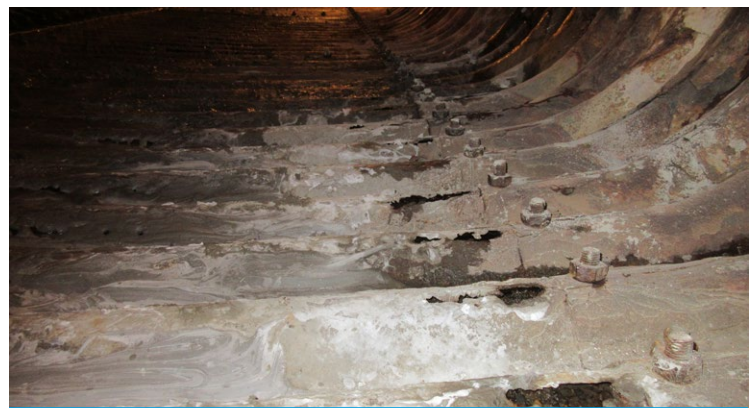
Filling of corrugations covering damage
