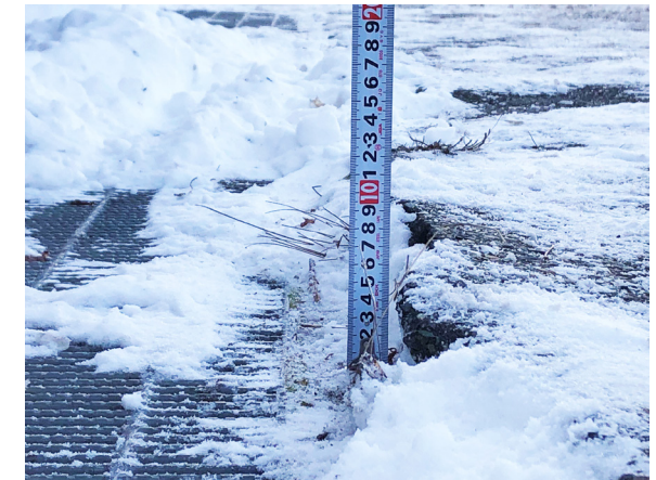
Pavement surface cracking due to frost action in subgrade
