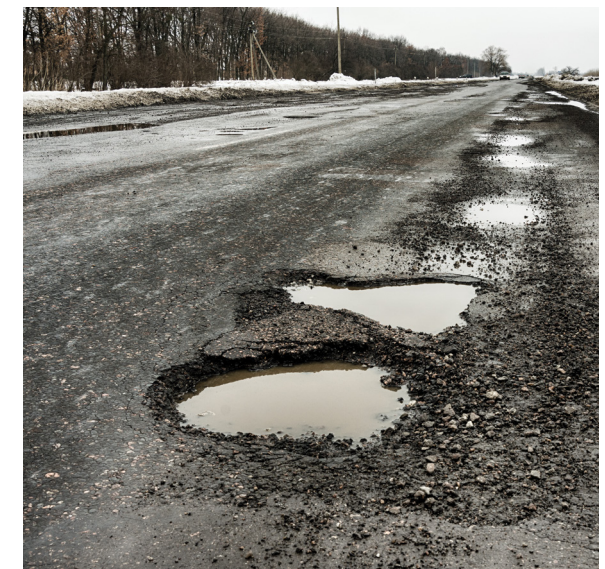
Frost boil through cracked pavement surface
