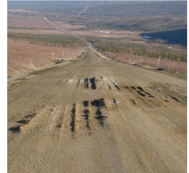
Basecourse rutting due to thaw weakened subgrade
