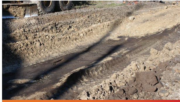
AN EXAMPLE OF SUBGRADE FAILURE
