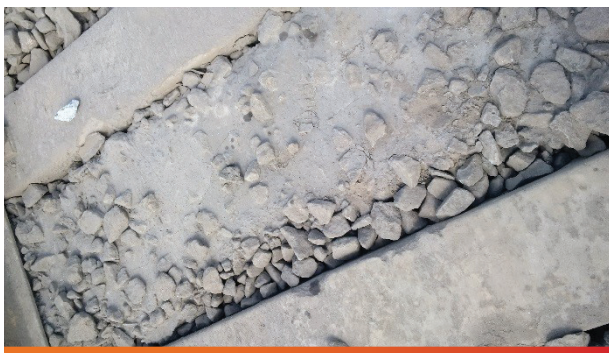
AN EXAMPLE OF BALLAST WITH PUMPING
