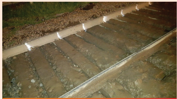
AN EXAMPLE OF MUD PUMPING FAILURE
